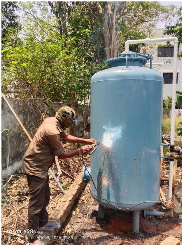
During: Welding work on the freshly painted blue carbon filter — new pipeline connections being fitted. The transformation from rust-red to clean blue is already dramatic.
