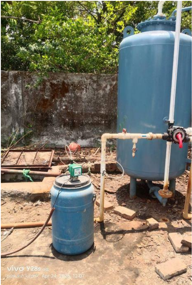
Culture dosing system — biological process restarted
