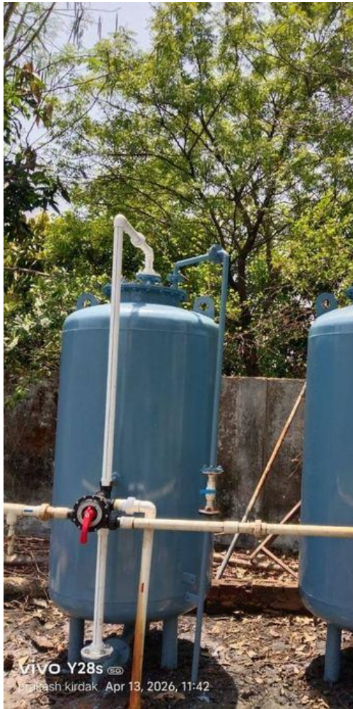
Twin filter vessels — fully painted, valved & commissioned
