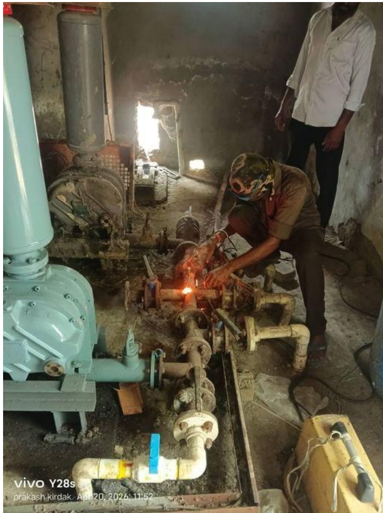
During: Inside the blower room — new lobe blower installed (left), technician welding the new pipeline manifold connections. This blower is essential for biological aeration.
