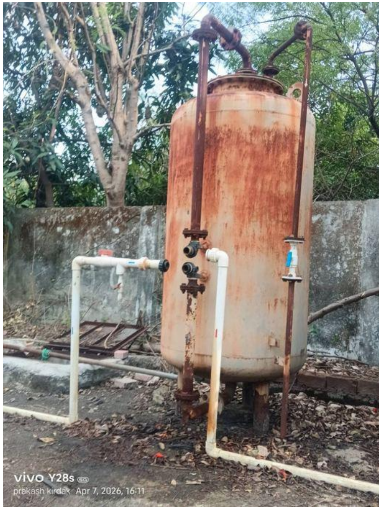
Before: Damaged pipeline connections and a severely corroded single filter vessel — structural integrity fully compromised
