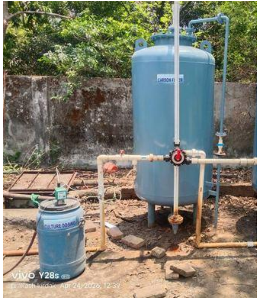
Sand & Carbon filters — ready for operation
