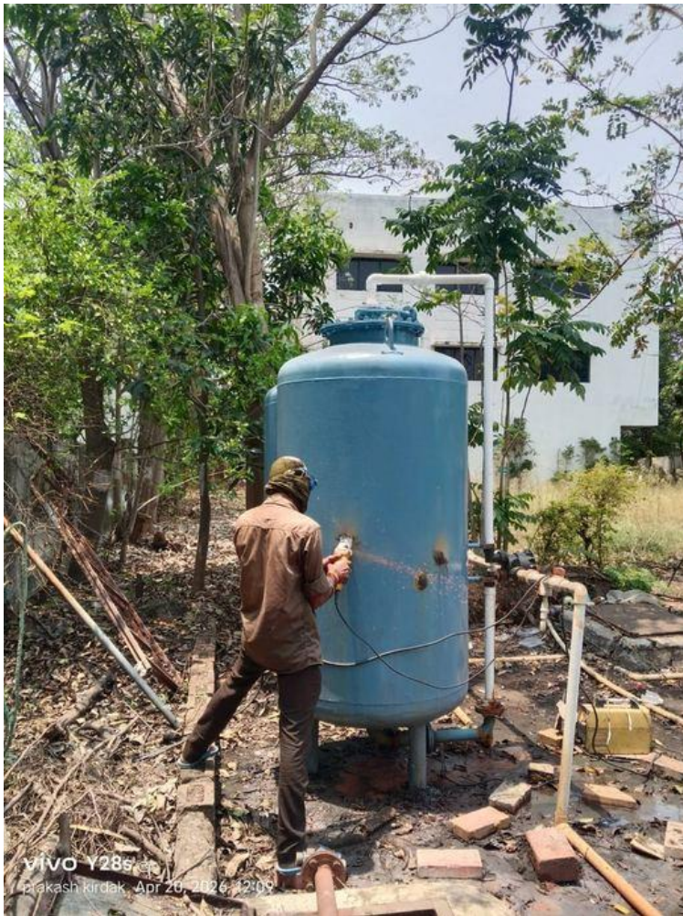
During: Angle grinding and surface preparation work on the second filter vessel — achieving the clean blue professional finish.
