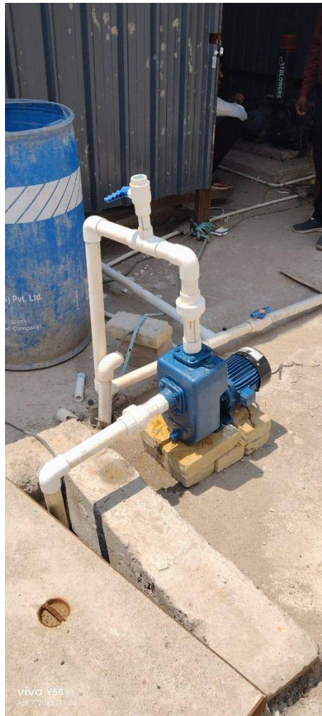
New collection tank pump installed — treated water can now be pumped for garden reuse
