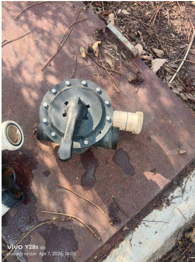
Before: The failed multiport valve — cracked and non-functional, lying on the ground. This single component failure cascaded into total plant shutdown.
