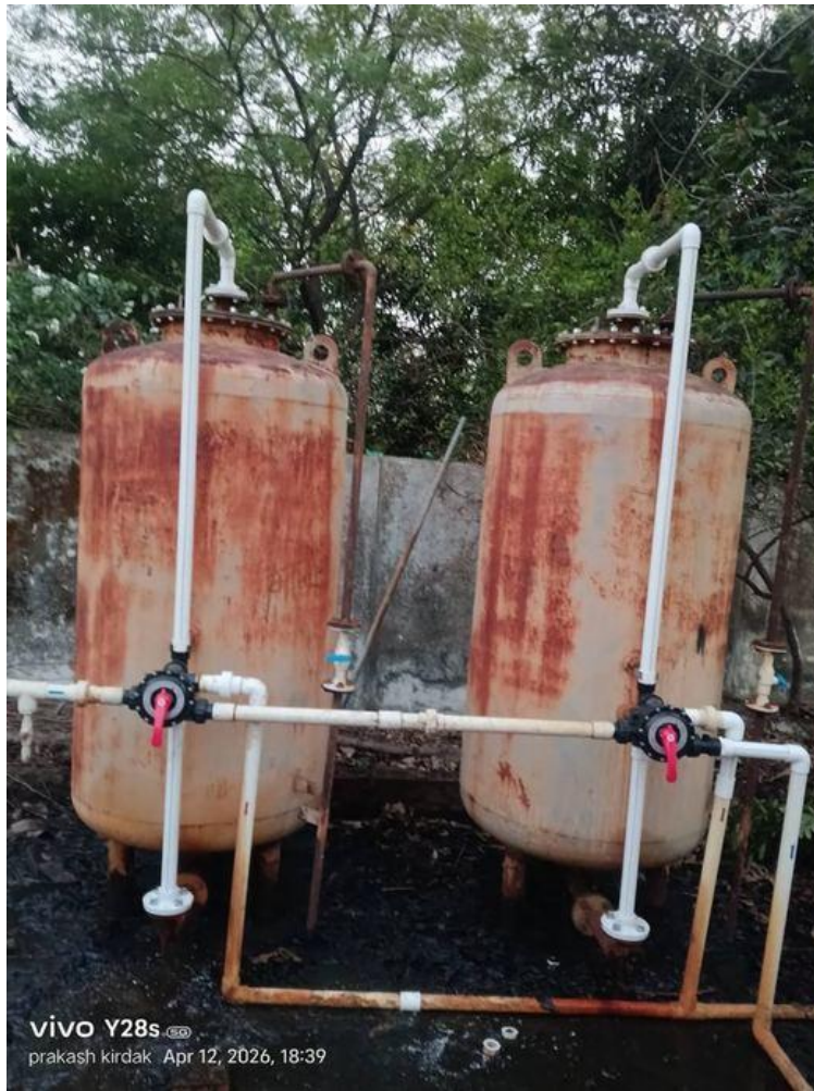
Before: Two heavily corroded MS sand filter vessels — 5 years of complete neglect, rust and waterlogged base
