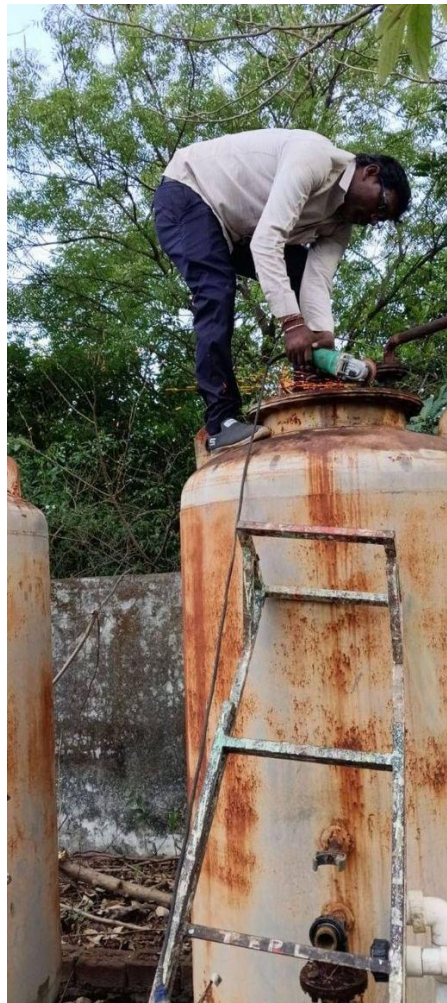
During: WCT technician on top of seized vessel — cutting open the backwash flange with an angle grinder. Sparks flying — this is the kind of hands-on skilled work most contractors avoid.
