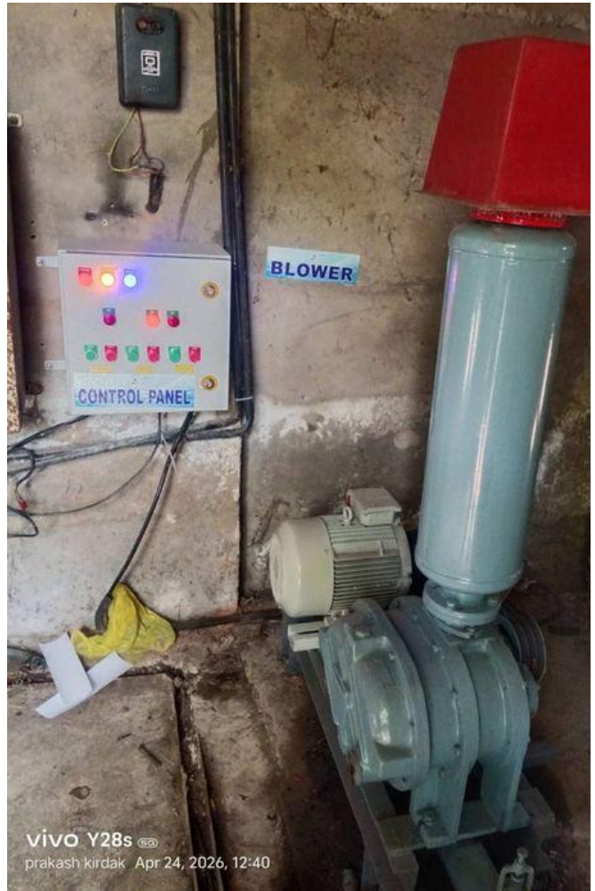
New control panel & blower — operational and labelled
