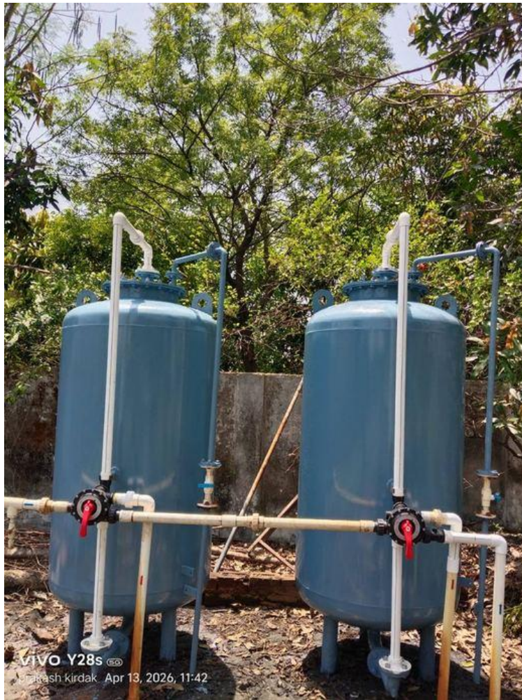
The complete STP — Carbon Filter + Sand Filter + Culture Dosing System — all fully operational and labelled. A professional installation. April 2026.
